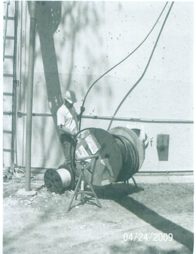
Andrew 7/8" hardline going up the tank.
